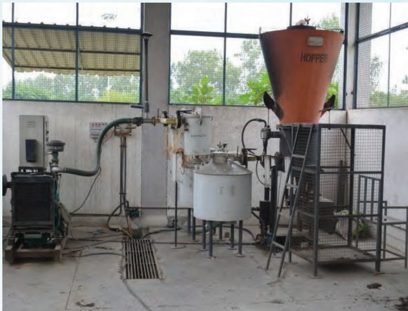
Biomass Gasifier Demo Plant (10 kW)
